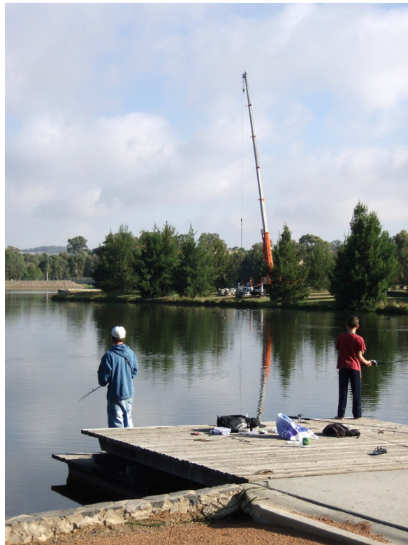
Crane lifting them in while a couple of local anglers observe carefully.
