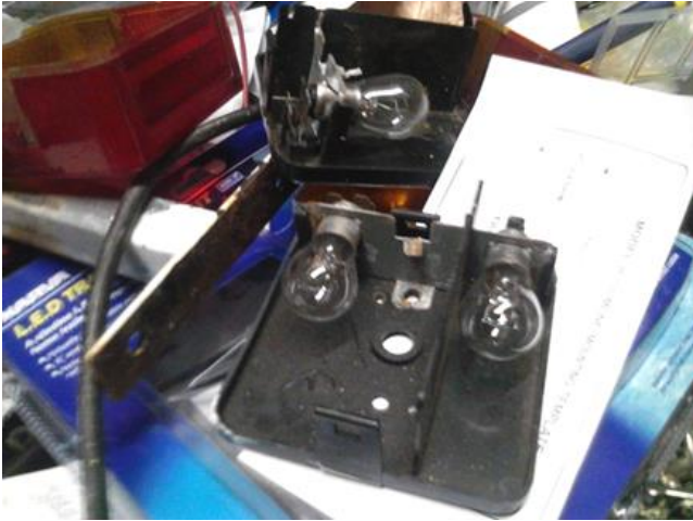
The old lights were rusted and not submersible
